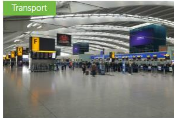
London Heathrow > LED lighting drivers, DALI control and emergency packs
